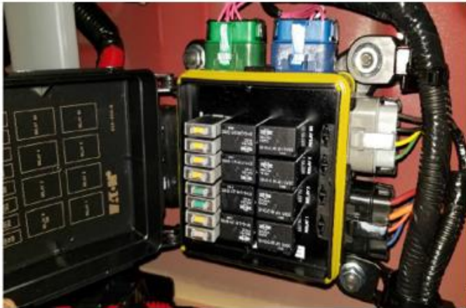
Figure 7.1.2.2: Overhead Switches dedicated electrical center
